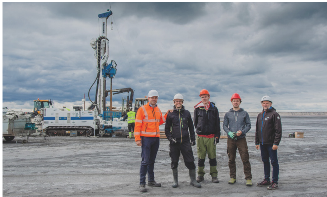
Ragn-Sells Project Manager Alar Saluste (left) with supporting research fellows in Estonia
